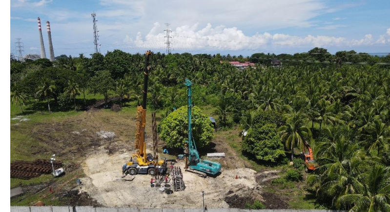
Top: NGCPs Sub station (May 2022)
